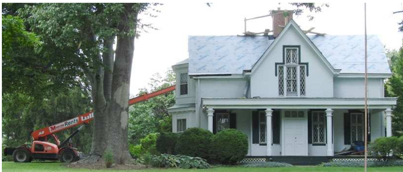
Progress at Tudor Hall on the Chimney Reconstruction and New Stainless Steel Roof August 25, 2009
